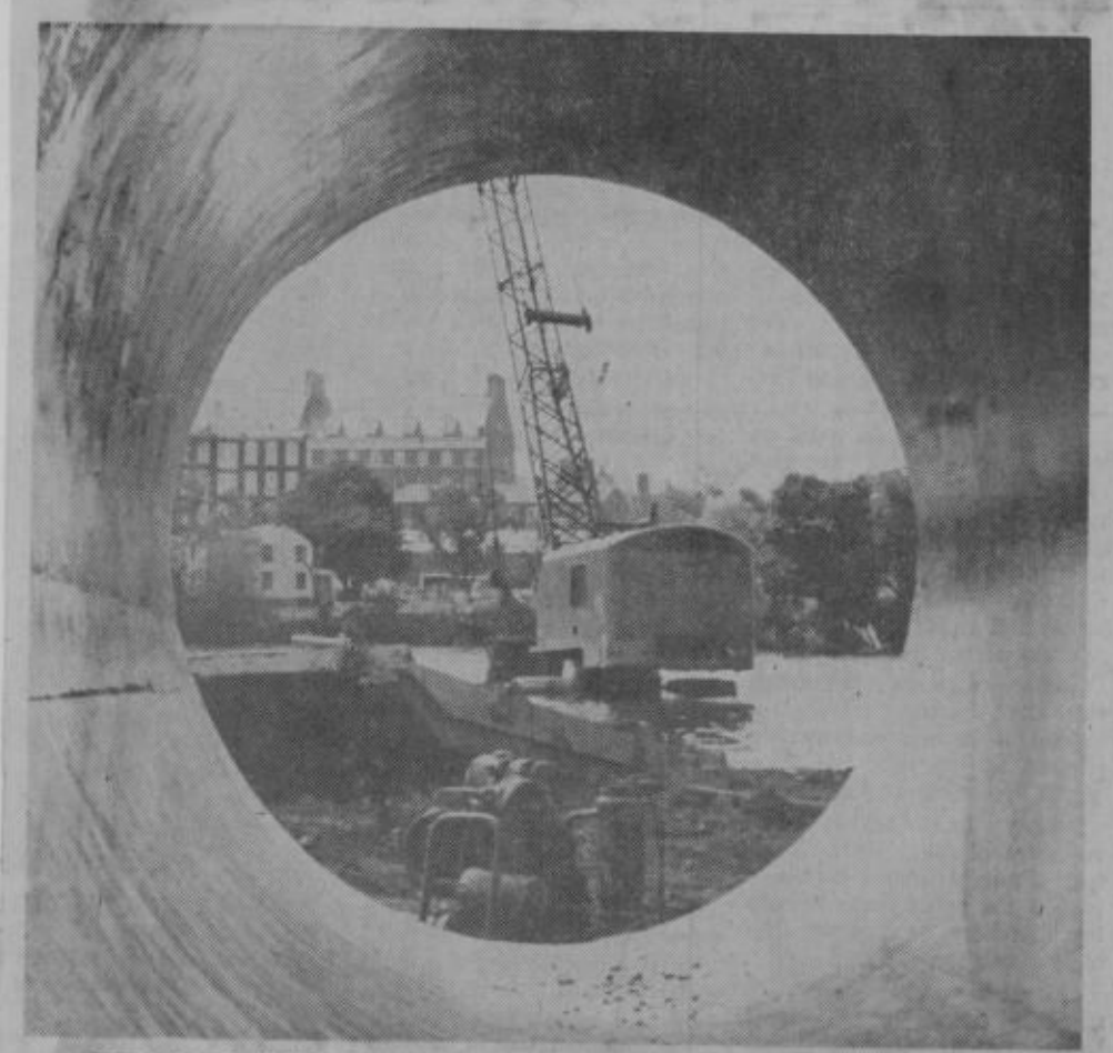
TARGET ON NEW BRUNSWICK — Workers place a 54-inch pipeline across the Raritan River to reach water in the Delaware and Raritan Canal. The project, undertaken by the Middlesex Water Co. of Woodbridge, would provide 20 million gallons a day in canal water for the company's customers. A section of the pipe above frames the Johnson and Johnson administration building.
