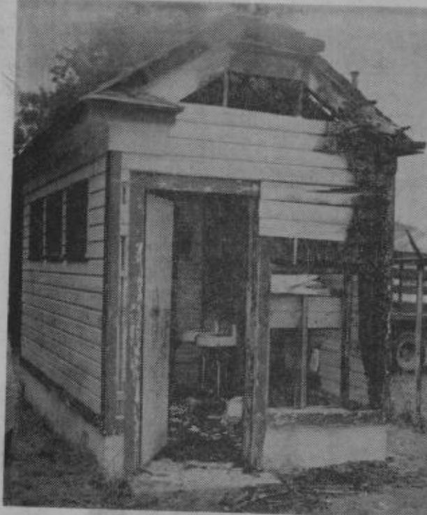
BEYOND REPAIR—A men's lavatory at Recreation Park was first burned. While boarded up pending repairs, vandals broke in and smashed toilet bowls
