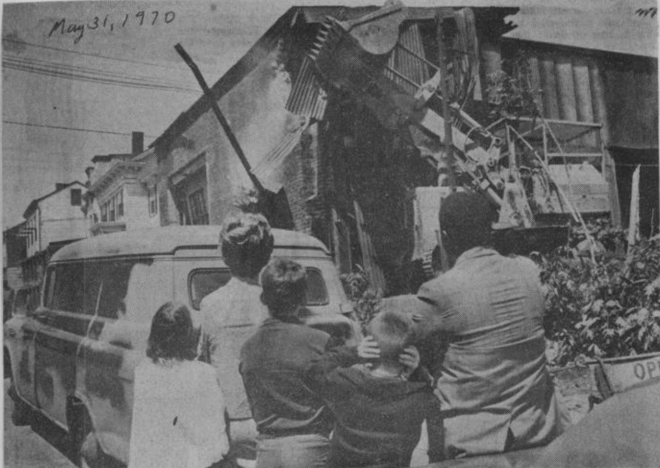
THE BIG SCOOP—A massive shovel tears into a building at Morris and Neilson Streets, marking the start of clearing buildings for the proposed George Street redevelopment program. Mayor Patricia Q. Sheehan, her three youngsters, Betsy, Danny and Mike (the noise was too much for the latter), and David Williams, New Brunswick Housing and Redevelopment Authority's assistant executive director, watch razing operation.
