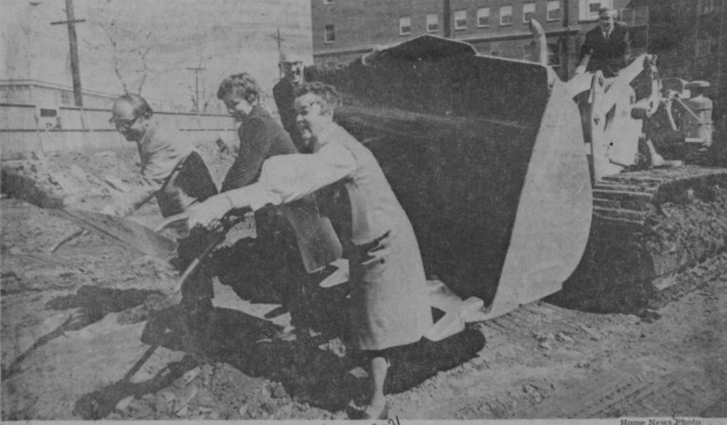
DIGGING IN — Hospital and city officials took up shovels and bulldozers yesterday to break ground for the Robert Wood Johnson Memorial Tower at Middlesex General Hospital. Holding shovels, from left, are Dr. Gabriel Pickar, deputy chief of staff, Mayor Patricia Q. Sheehan and Sister Joan Manion, administrator of St. Peter's General Hospital. Edwin Baier, chairman of Middlesex Board of Directors, sits in driver's seat, while Joseph Henry, hospital president, looks on.
