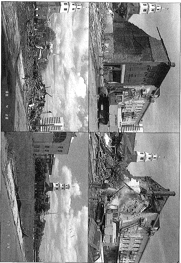
Figs. 6–9. These photographs document the demolition of the Phoenix Engine Company on Dennis Street in New Brunswick's Hiram Market Historic District in April 1988. By 1992 the section of the historic district along Dennis Street had been completely cleared in preparation for a townhouse/condominium development. The original Hiram Market house stood in front of the Reformed Church, on the left in the last photograph.
